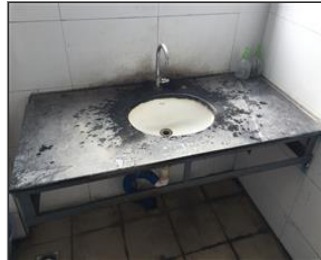
Photo of non-conformity 5-3 Photo of dirty washing facility.JPG
