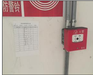
Photo of fire safety equipment 4-6 Photo of fire alarm.JPG
