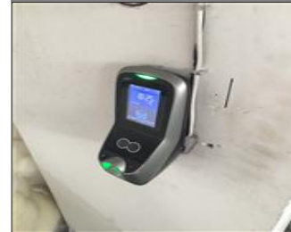
Photo of the inside of the main production hall 14-4 Photo of attendance recorder.JPG
