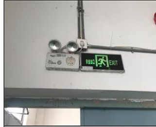
Photo of fire safety equipment 4-3 Photo of emergency lights exit indicator.JPG
