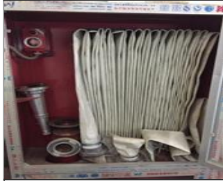
Photo of fire safety equipment 4-2 Photo of fire hydrant.JPG
