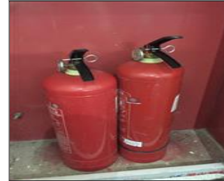
Photo of fire safety equipment 4-1 Photo of fire extinguishers.JPG
