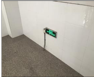
Photo of fire safety equipment 4-5 Photo of exit route with marking.JPG
